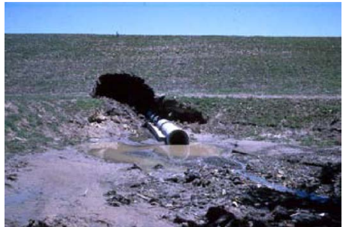
Photo 4: Piping failure along outlet conduit
