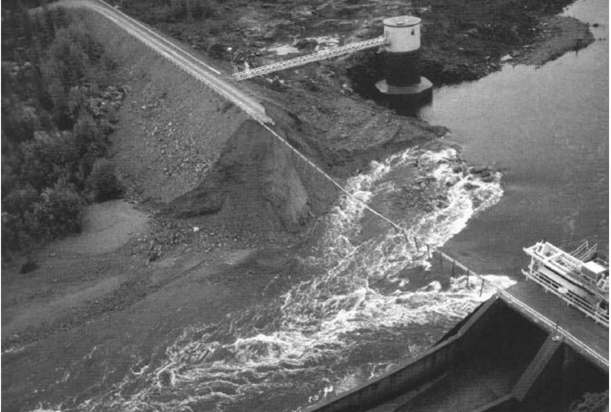
Breach of Noppikoski Dam on September 7, 1985
