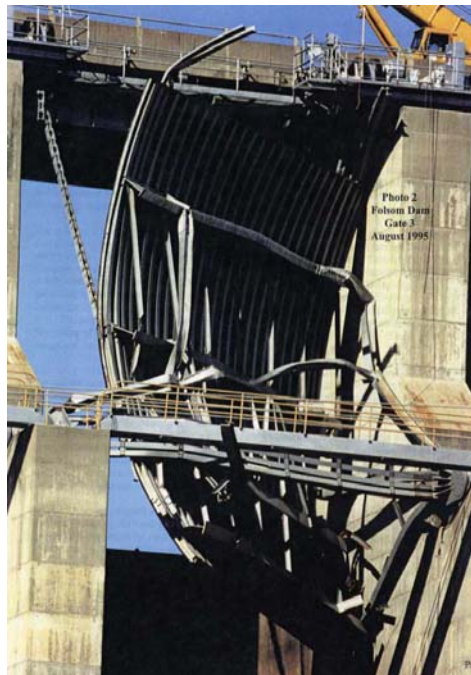
Figure 30-1 – Folsom Dam Radial Gate Failure
