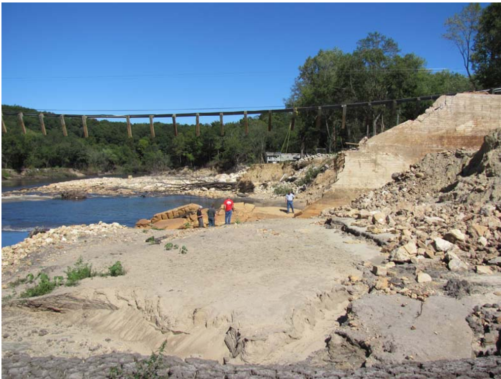
Figure 7. IPE investigation of former embankment foundation. Remnants of core wall on the right side of photo. Source: Iowa DNR
