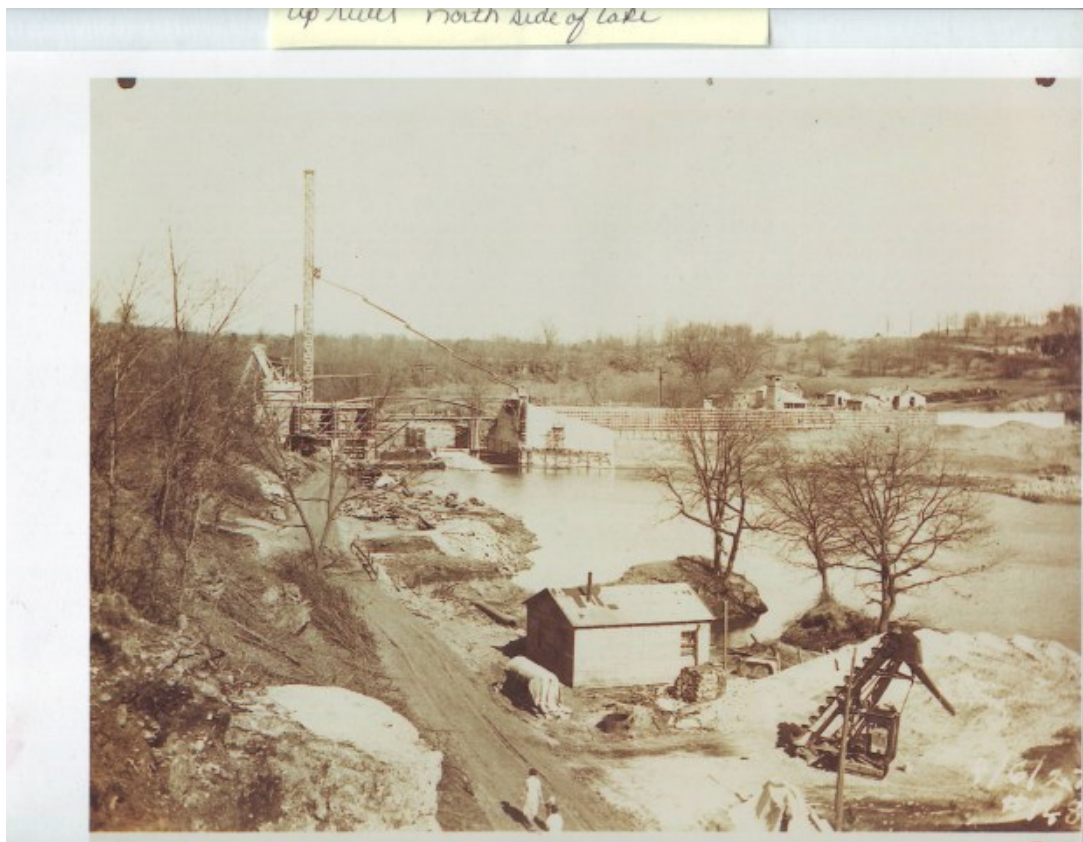
Figure 2. Construction of the dam. Core wall construction shown on the right end. Source: LDRA
