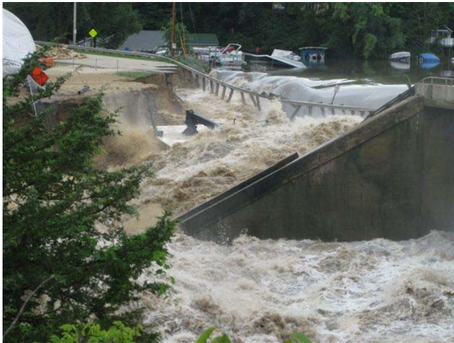
Figure 12. Breach in progress, core wall still in place. Source: Iowa DNR.
