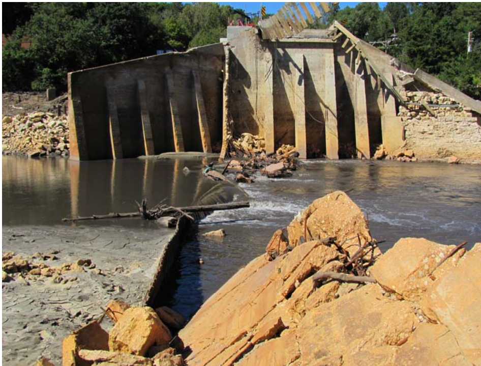
Figure 8. Remnants of sheet pile, core wall and spillway wingwalls. Source: Iowa DNR
