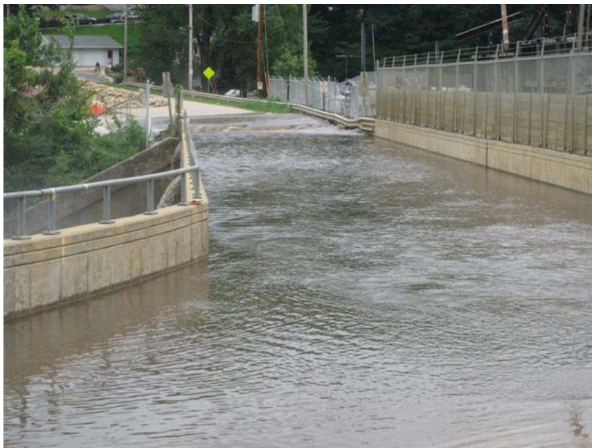
Figure 10. Breach in progress, headcut completely through roadway. Source: Iowa DNR.
