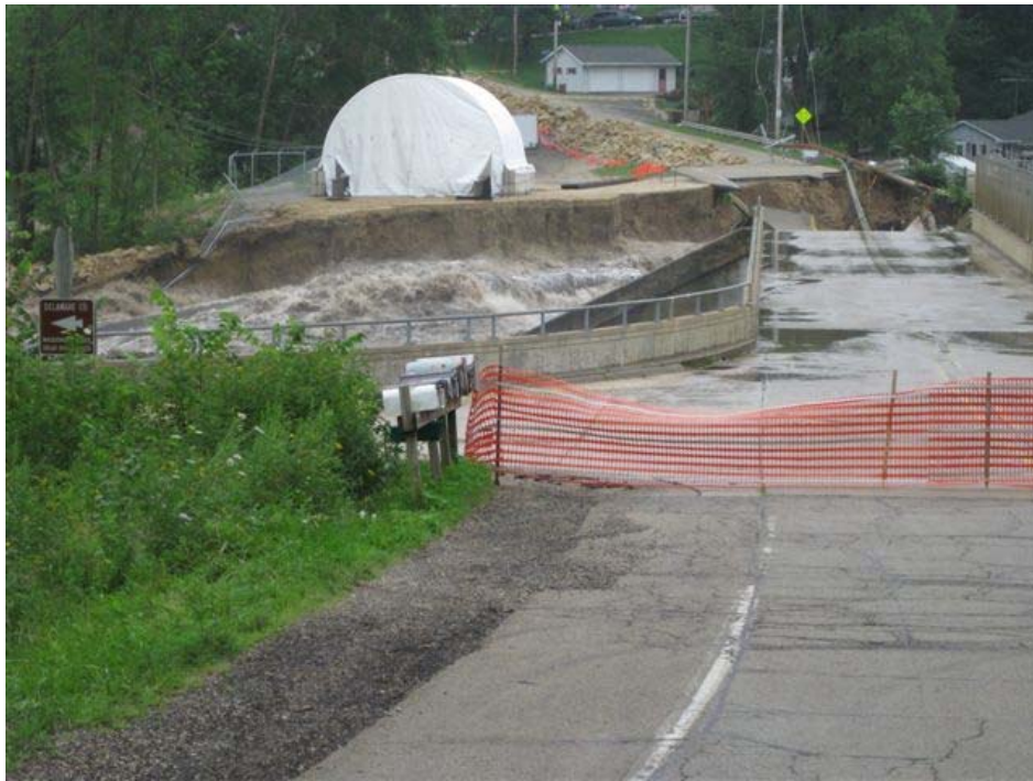
Figure 13. Full breach and uncontrolled release of water. Source: Iowa DNR.
