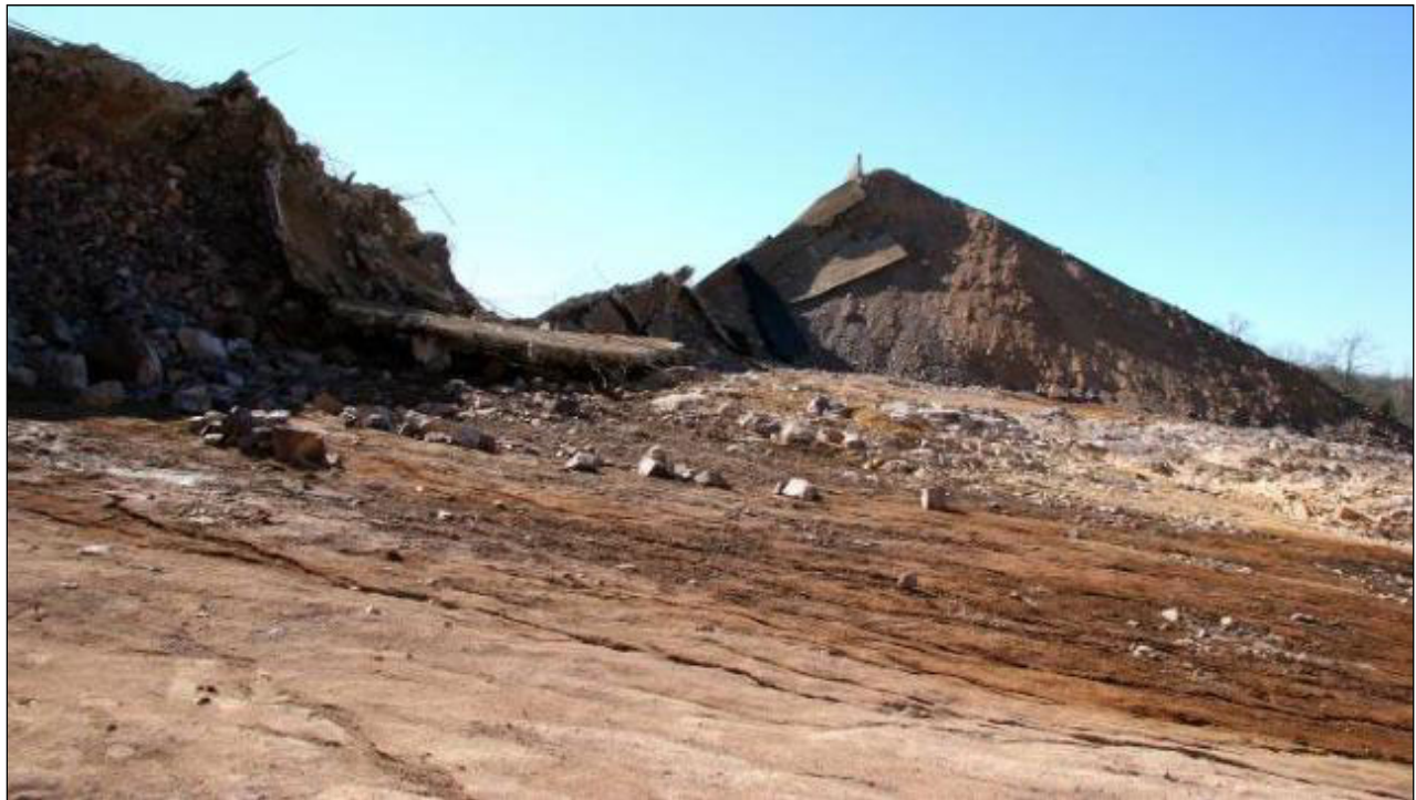
Fig. 18. – The remnant lip as seen at the failure site.
