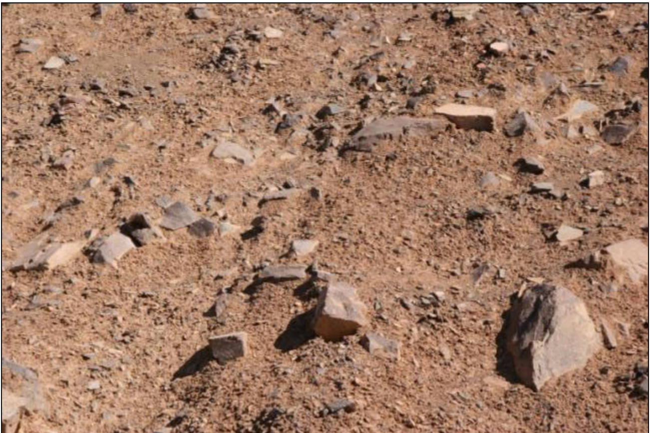
Fig. 19. - Close up of "dirty" rockfill exposed on lateral margins of the breach. The large clasts are 10-12 inches diameter.
