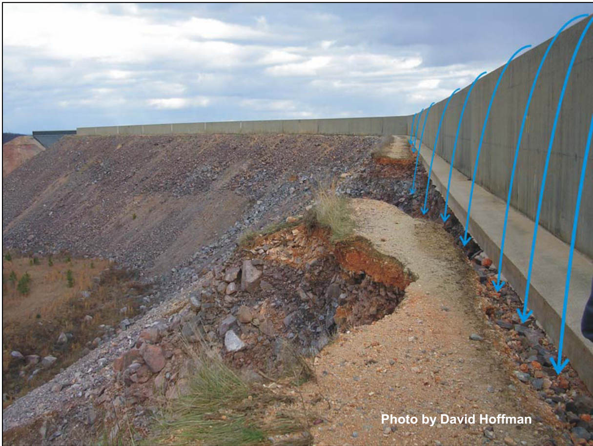
Fig 9. – This photograph shows arrows representing the overflow nappe once it extended beyond the 3 foot wide wall footing and directly onto the underlying rockfill. The rate of scour and erosion increased dramatically once this occurred.
