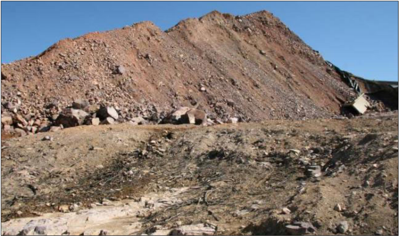
Fig. 21. – Residual soils, including tree roots and other organic matter, were observed left in place beneath the failed portion of the upper reservoir embankment.
