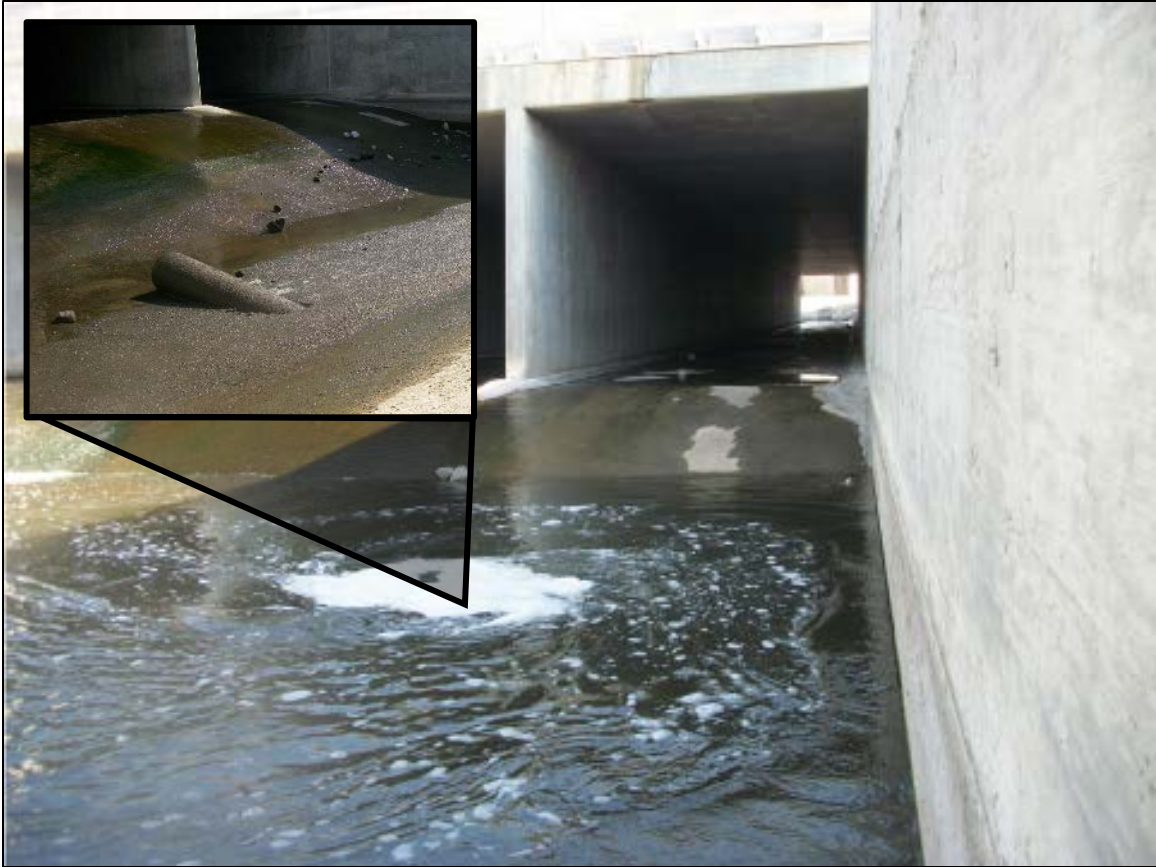
Figure 7. Photograph showing inlet pipe at Lake Wanahoo Dam where boy became trapped and drowned. Photographs courtesy of Tim Gokie.
