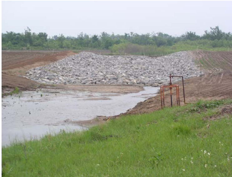
Figure 6. Rock chute spillway on Little Washita Site 13 in Grady County, OK (photo courtesy Chris Stoner, USDA-NRCS).
