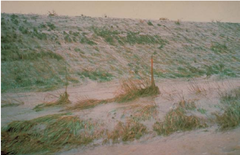
Figure 4. Vegetated embankment experiencing overtopping flow.
