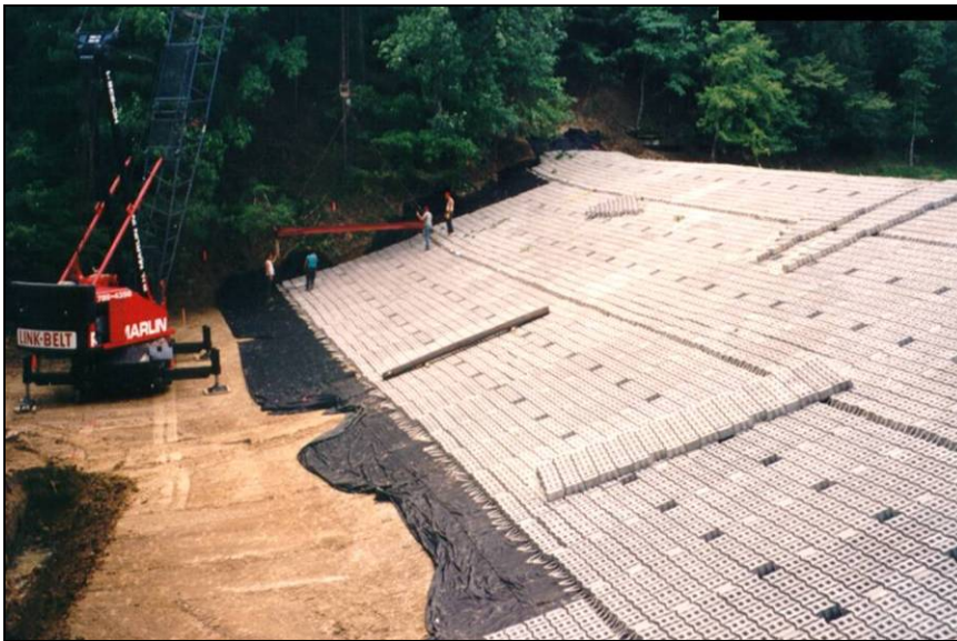
Figure 3. Placement of cable-tied mats over a geotextile on the downstream face of Strahl Lake Dam, Indiana (Photo by Contech Construction Products, Inc.)
