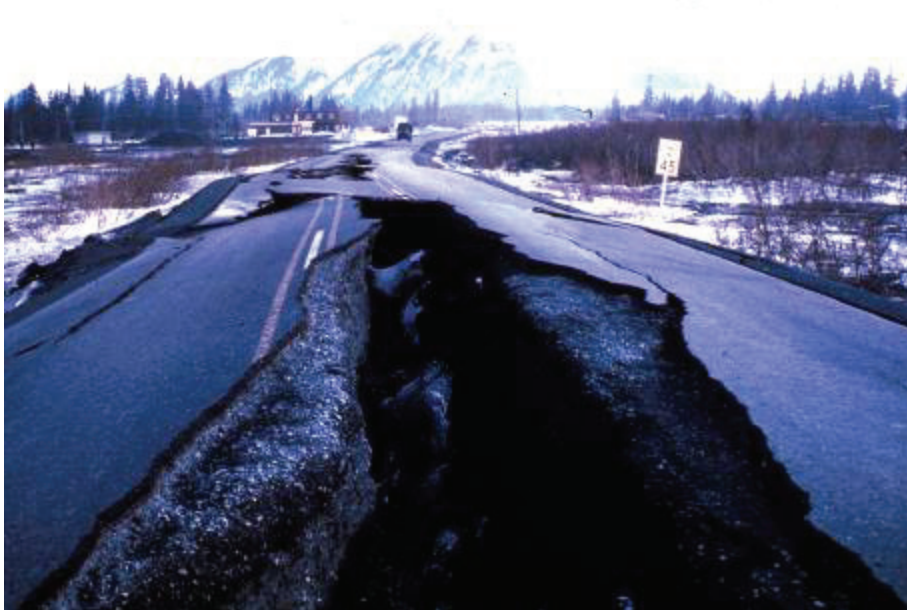
Figure 6-2 Roadway damage from the 1964 Alaska earthquake (Photo from United States Geological Survey).
