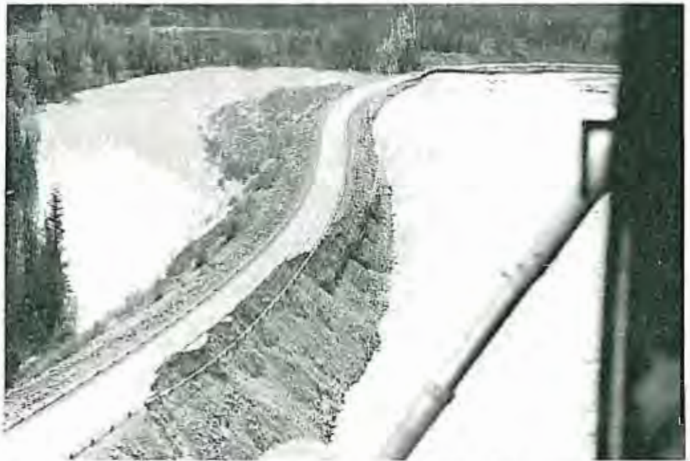
Flooding water from the Middle Fork of the Flathead River washed fill away and undercut a new section of Highway 2 at Nyack between Essex and West Glacier. Guest photo.
