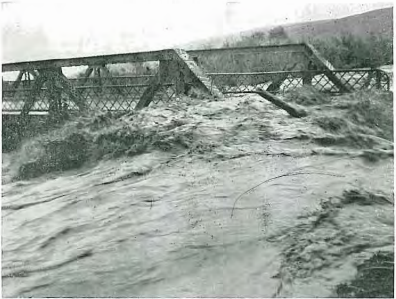
Muddy Kennedy Creek north of Babb on Highway 89 is in full flood as it carries tons of debris over the approach road to this steel bridge. The bridge dropped into the river bed finally. George Goggins photo.
