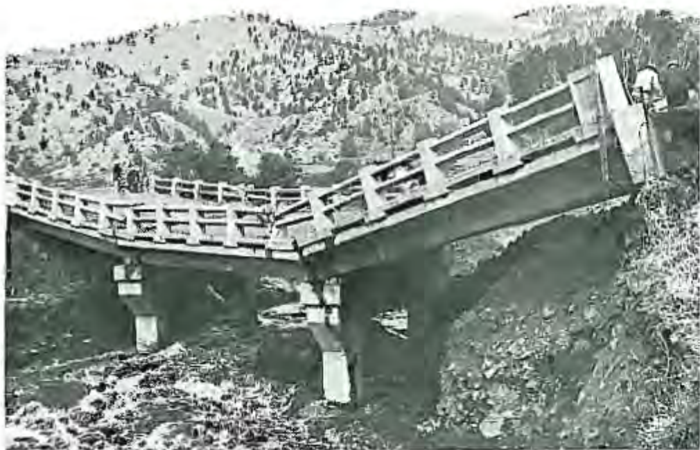
One of the most important bridges to go out during the central Montana flood was the structure over Hardy Creek on U.S. 91 between Great Falls and the capital city of Helena. Motorists had to detour over 7,389-foot Kings Hill Pass to reach Great Falls from Helena, Len Ashburn photo.
