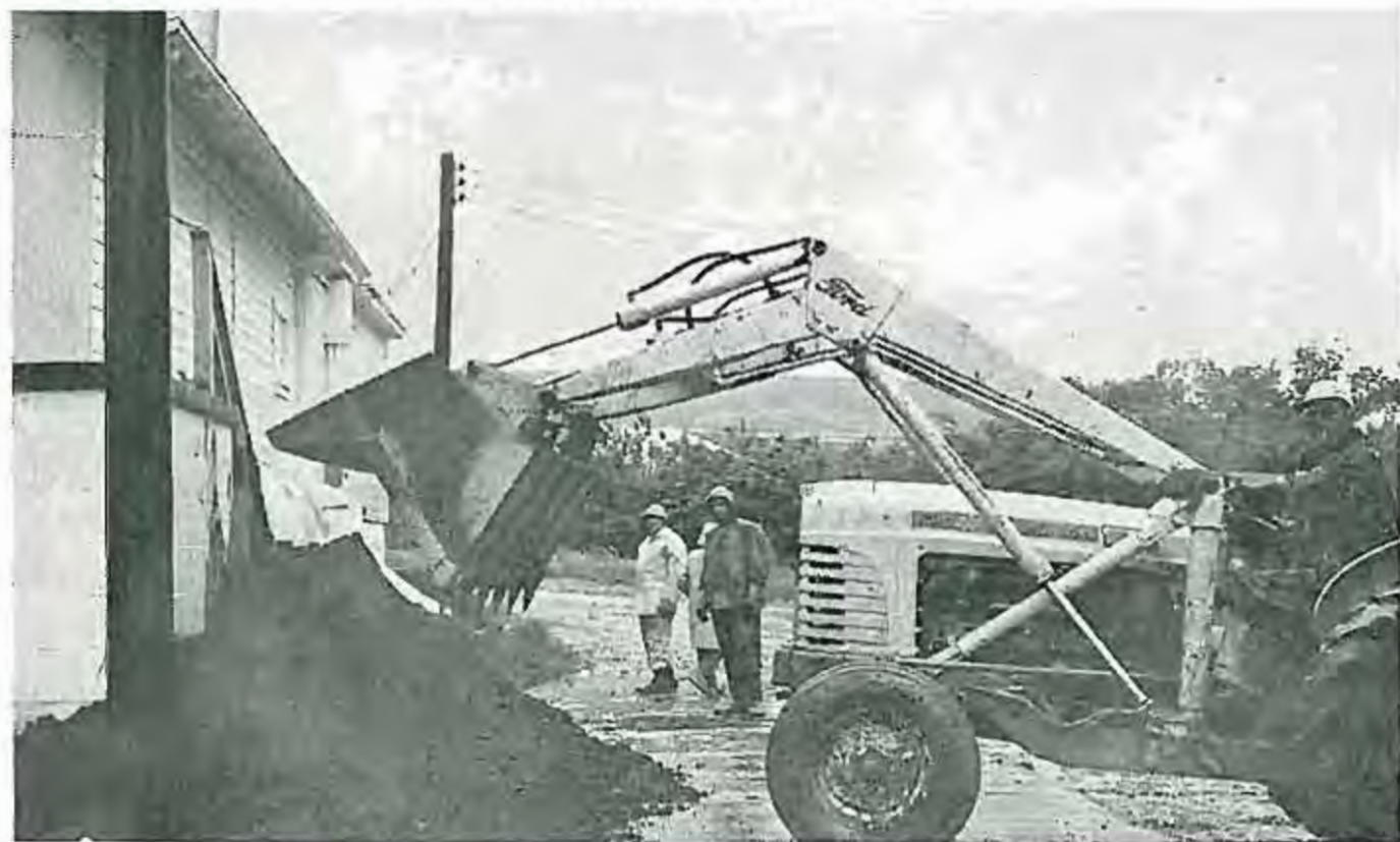
The Beacon Bar on the old Sun River road between the Sixth Street Southwest and Fourteenth Street Southwest bridges got pre-flood protection from sheets of plastic secured against the building with dirt piled against them. Tribune photo.
