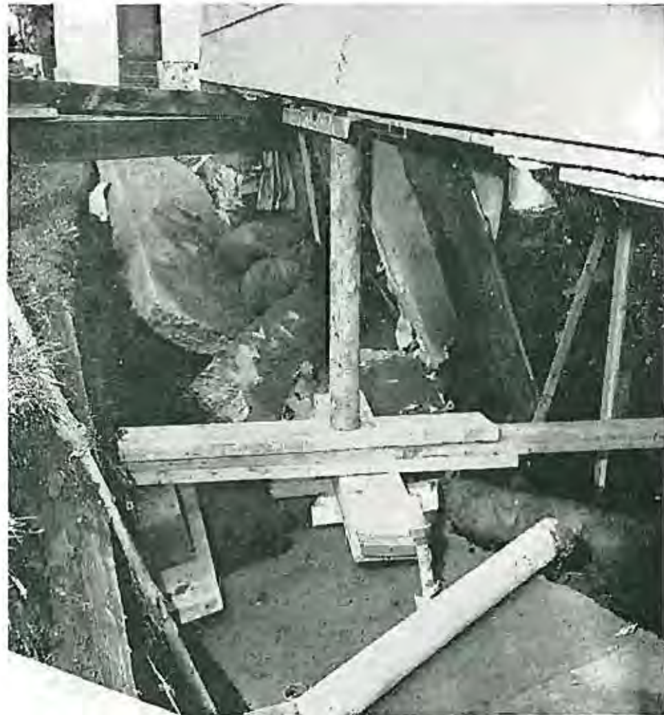
The flood left a major rebuilding problem at the Great Falls home of William J. Burton, 2125 4th Ave. SW. Terrific pressure of Sun River floodwaters buckled the concrete wall of this section of the basement, opening up the back of the house. Timbers were thrust through the hole and out a basement window on the other side of the house to support the weight of the structure at that point. The house is owned by Ira McFadden. Tribune photo.
