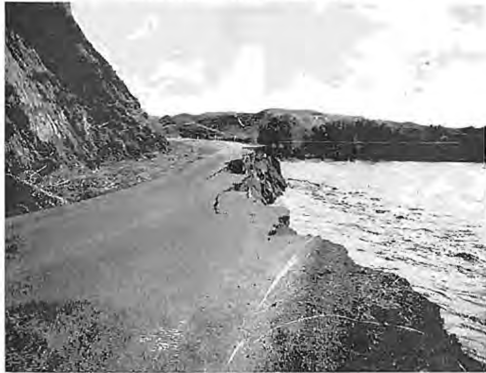
The rampaging Teton River washed out this section of Highway 87 about five miles north of Fort Benton when the flood crest hit. This view shows little more than a footpath remaining of the once-wide thoroughfare. John Saks photo.
