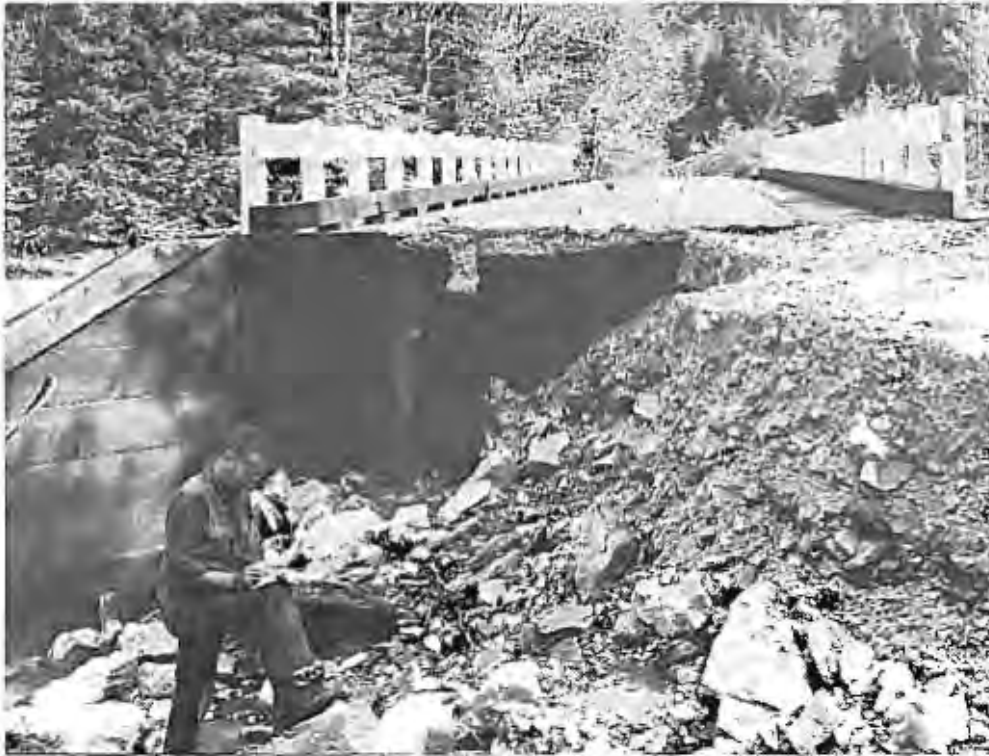
Dave Terry, Forest Service, inspects the flood-damaged Windy Ford bridge over the South Fork of the Teton River. Forest Service photo.
