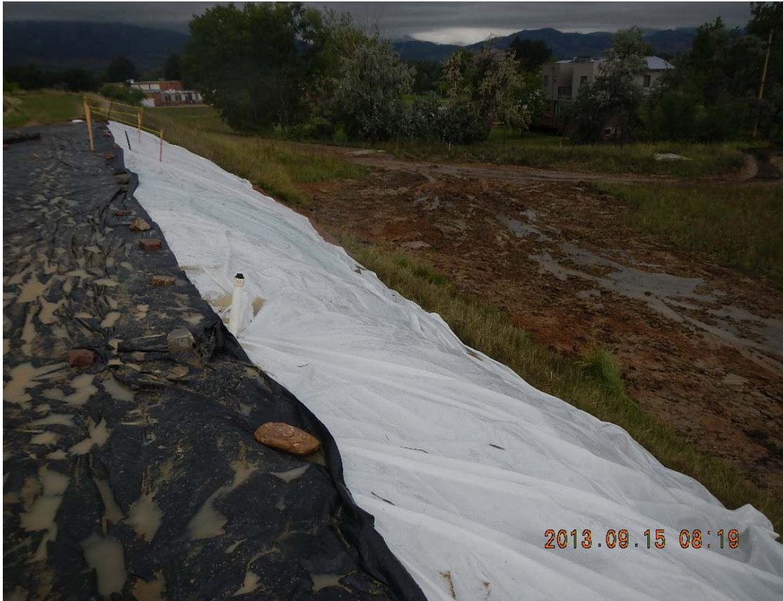
Figure 7 - Temporary stabilization measures along the reach of the downstream slope that had sloughed at Baseline dam.
