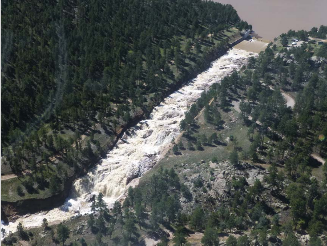
Figure 13 - Button Rock dam spillway flows from the air on September 16, 2013.
