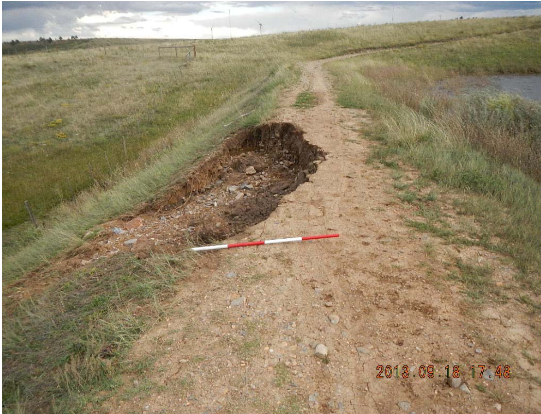
Figure 16 - Photo of a slope failure caused by embankment saturation due to overtopping of the Flatirons Vista dam. The weakened dam was eventually breached.
