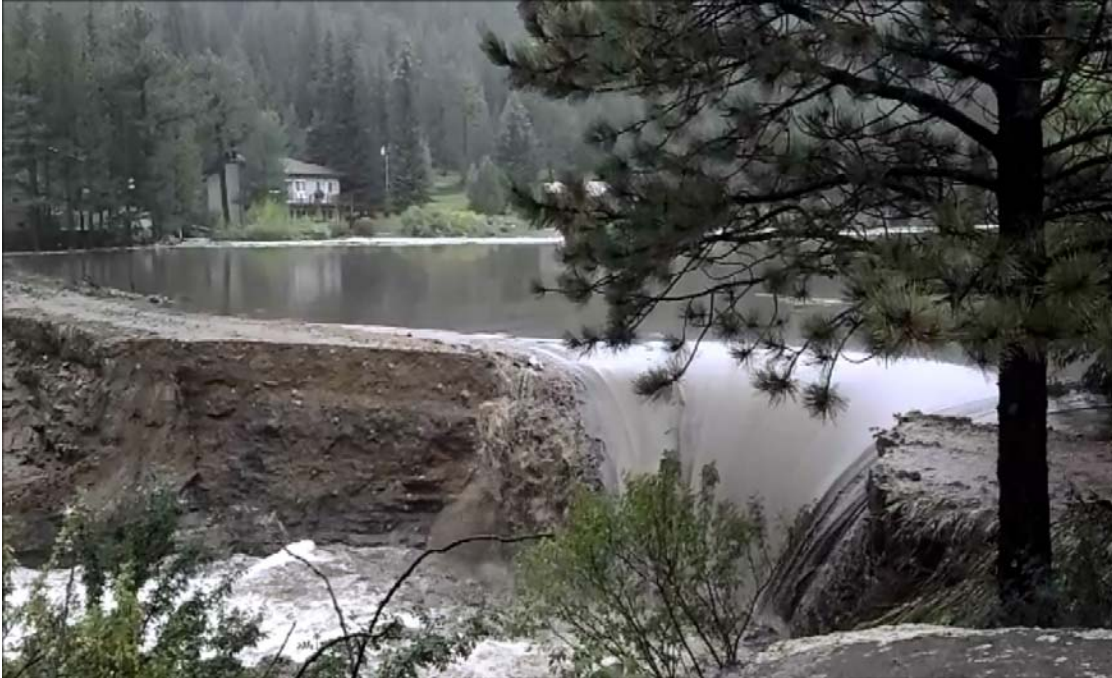
Figure 4 - Photo of Meadow Lake dam as the full breach develops at 1:40 P.M. on Thursday September 12.
