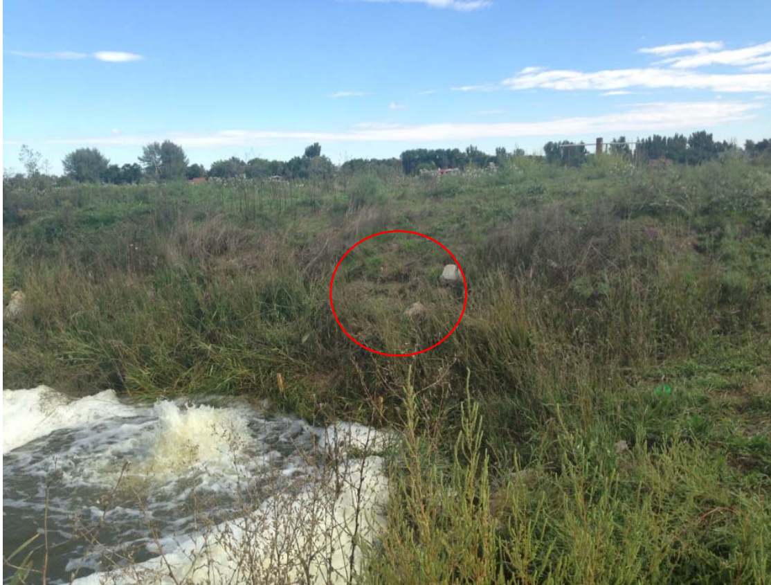
Figure 14 - Photo of the swollen outlet channel at Gaynor Lake dam. Note location of sinkhole above the pipe.
