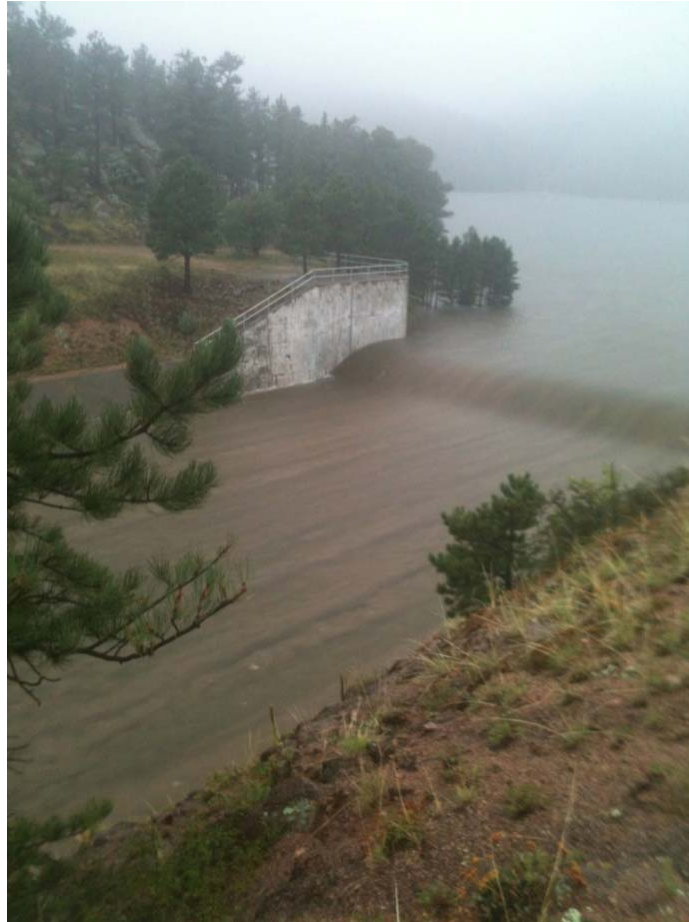
Figure 12 - Photo of Button Rock dam spillway flow from the left abutment, near peak (10,000 cfs) on Friday September 13, 2013.
