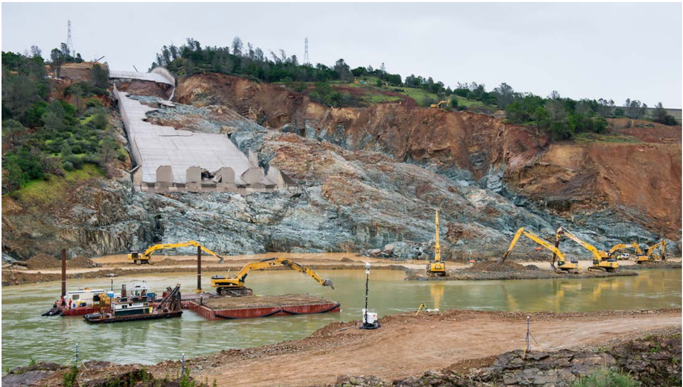
Figure 7. Debris removal in the diversion pool below Oroville Dam with the damaged principal spillway in the background. (Photo courtesy of CA DWR).
