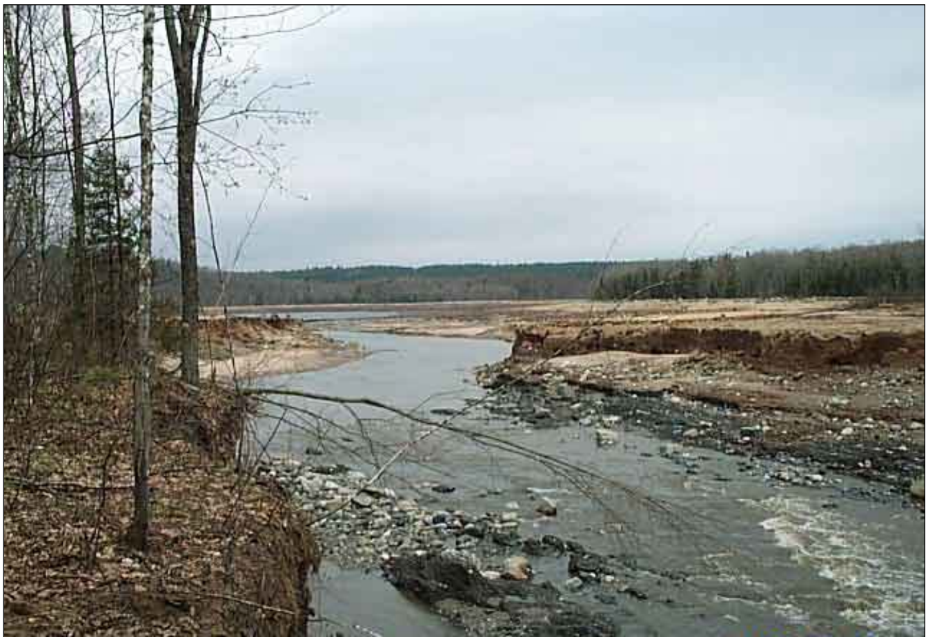
Figure 1. Channel cut through the Silver Lake Dam emergency spillway, looking upstream (Photo courtesy of FERC)
