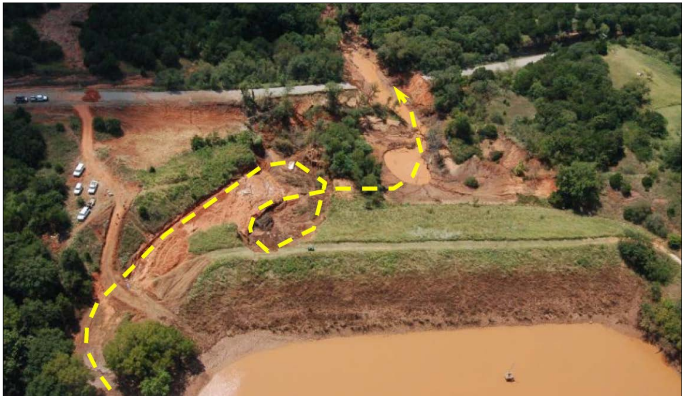
Figure 6. Photograph showing the flow path and erosion in the downstream slope of Sugar Creek Dam in Caddo County, Oklahoma (Photo courtesy of Danny McCook).
