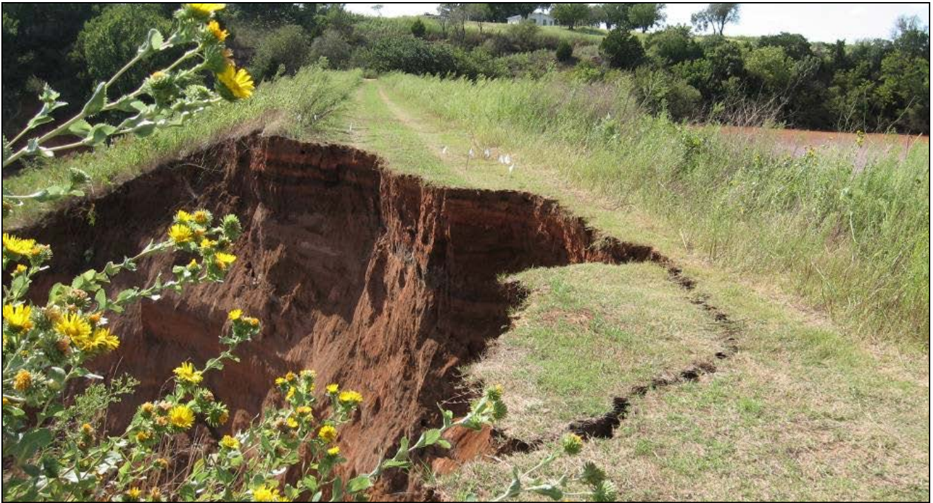
Figure 5. Photograph showing the erosion in the downstream slope of Sugar Creek Dam in Caddo County, Oklahoma (Photo courtesy of Danny McCook).
