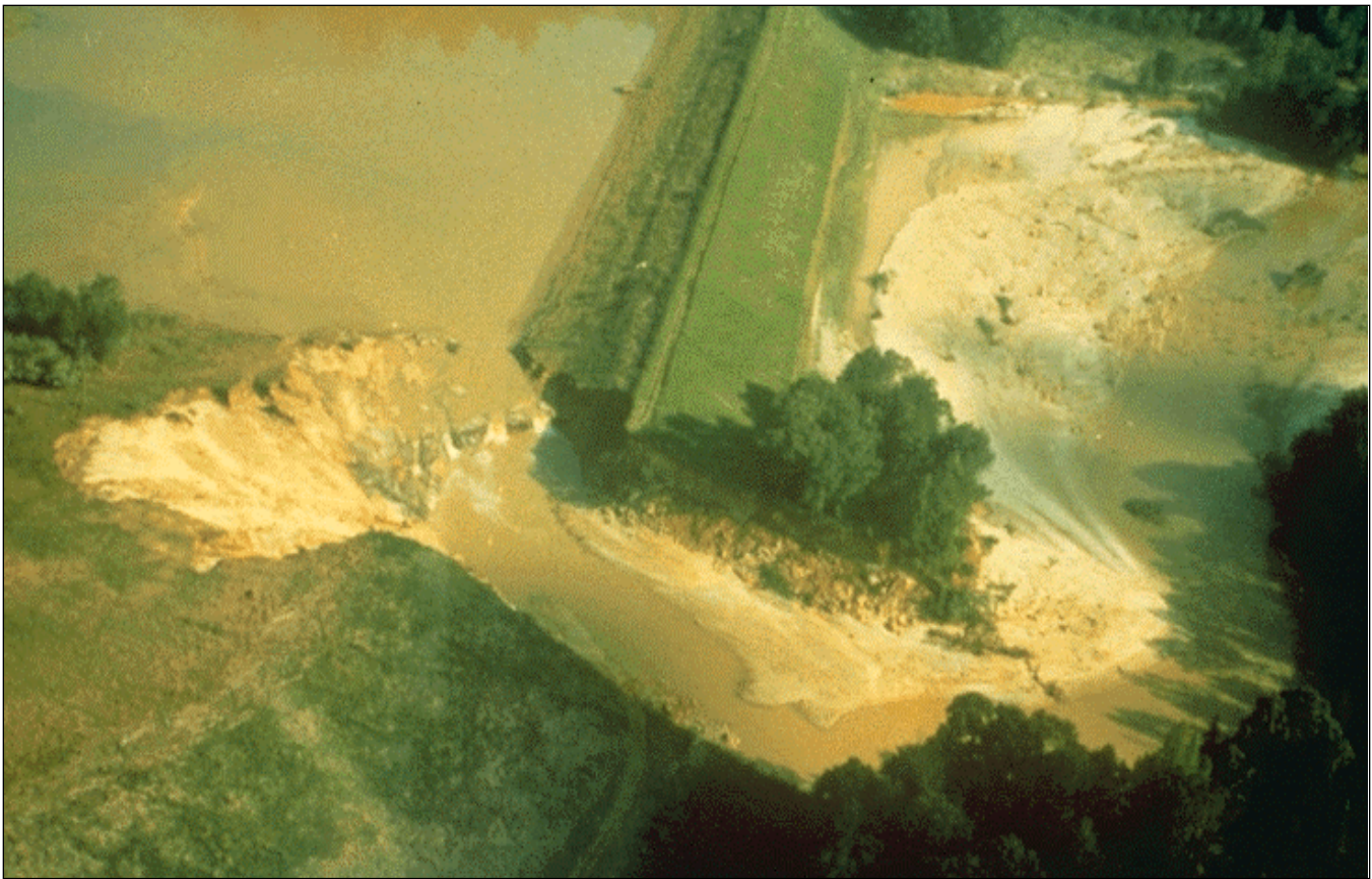
Figure 4. Overview of the failed auxiliary spillway at Black Creek No. 53 Dam (Photo courtesy of Darrell Temple).
