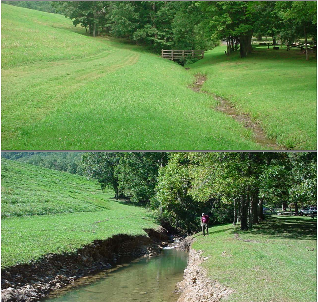
Figure 2. Auxiliary spillway discharge channel before (TOP) and after (BOTTOM) initial activation of the spillway, looking upstream (Photos courtesy of Tom Roberts, VA DCR)
