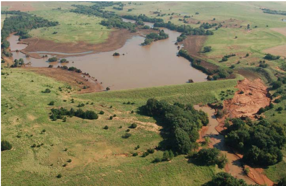
The auxiliary spillway of Sugar Creek Watershed Dam No. L-43 was damaged in August 2007, when the dam's watershed received 8.3+ inches of rain in a 6-hour period.
