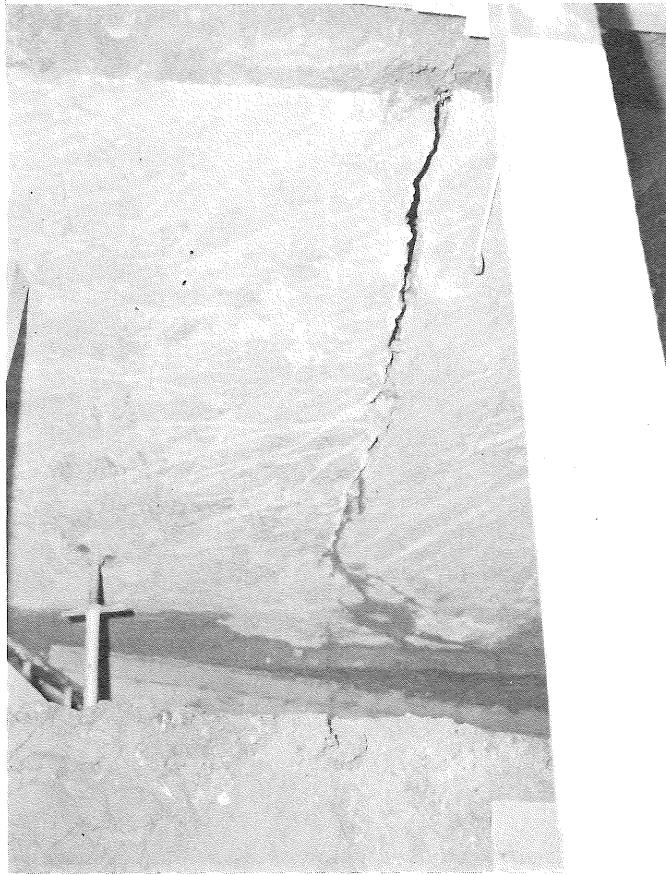
PHOTO 77. Break in north wall of drainage inspection chamber at Station 0+70.3, as exposed in Excavation No. 7B.
