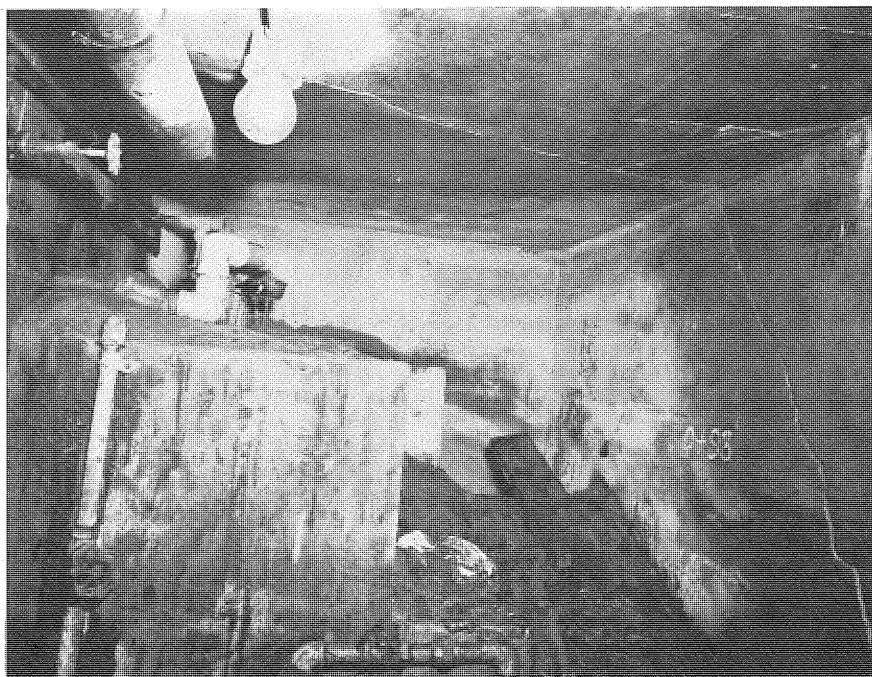
PHOTO 73. West end of drainage inspection chamber, showing crack at Station 0+89, drains, and weir box, December 20, 1963
