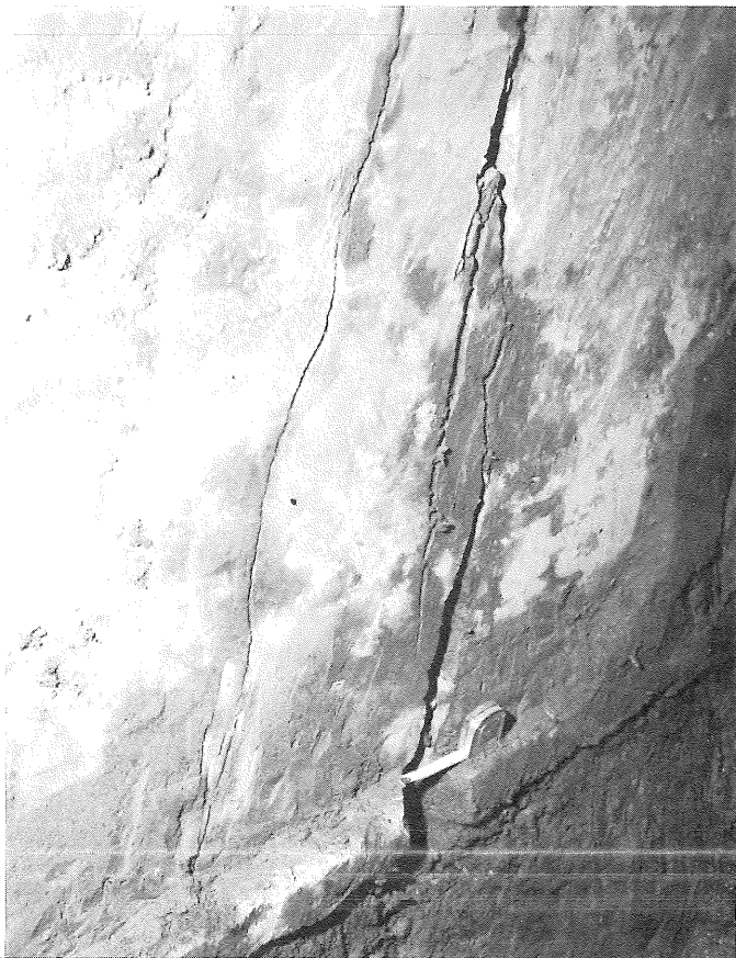
PHOTO 80. Bottom of break in north wall of drainage inspection chamber of Station 0+89.
