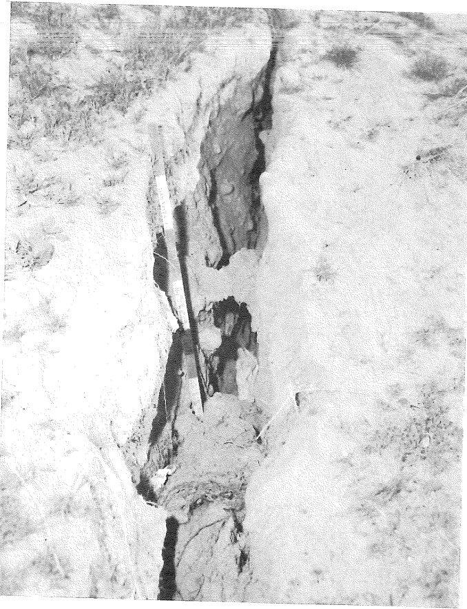
PHOTO 57. Earthcrack 9. Looking north showing open crack near base of slope northwest of detention basin and south of Cloverdale Avenue.
