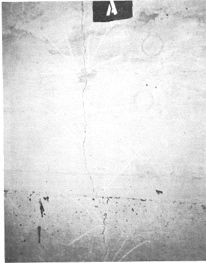
PHOTO 51. Crack in drainage inspection chamber at Station 0+70.3, January 10, 1952.
