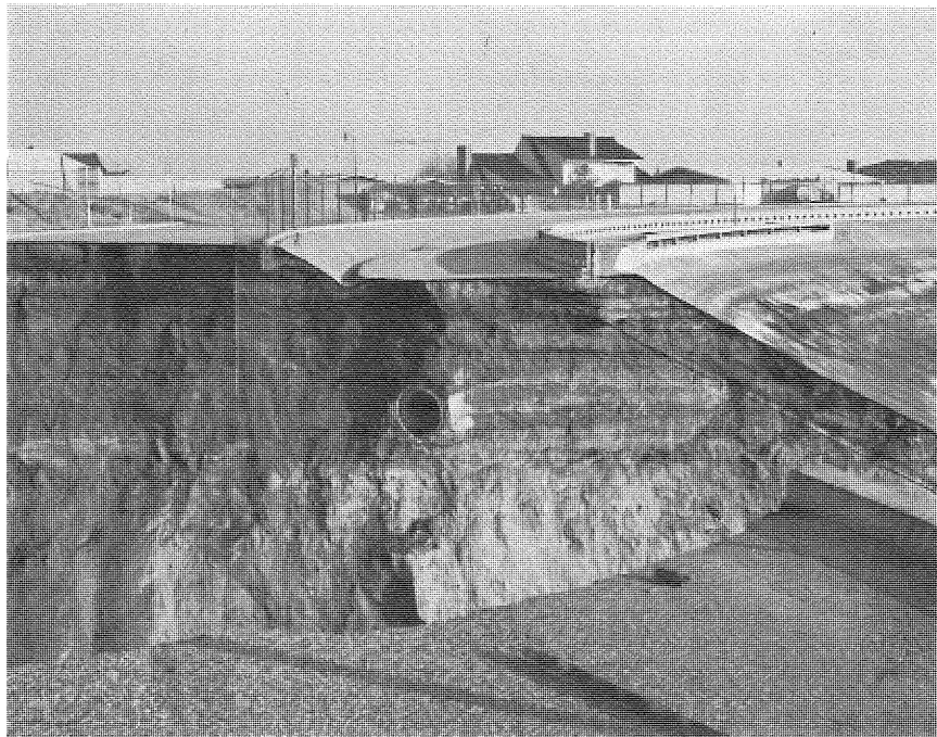
PHOTO 71. East side of breach showing spillway pipe and reservoir lining, December 22, 1963.
