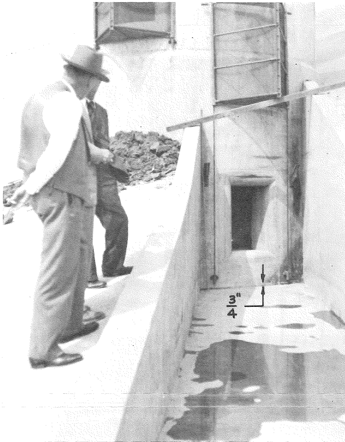
PHOTO 50. Settlement of gate approach channel, May 11, 1951
