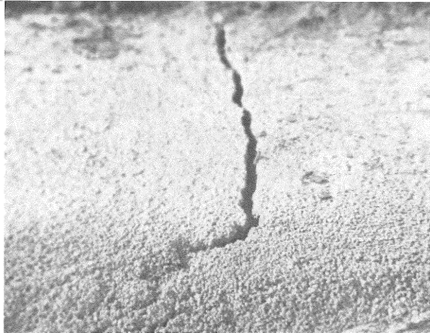
PHOTO 40. Crack in 4-inch cemented pea gravel discovered during construction.
