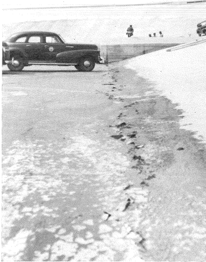
PHOTO 49. Buckling of asphaltic paving, May 11, 1951.
