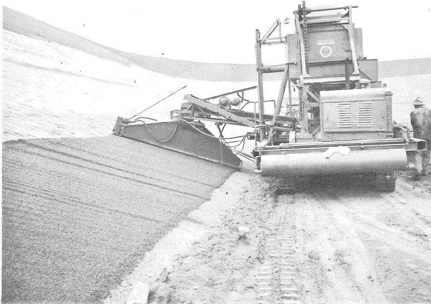
PHOTO 35. Kemper pea-gravel slope spreader.
