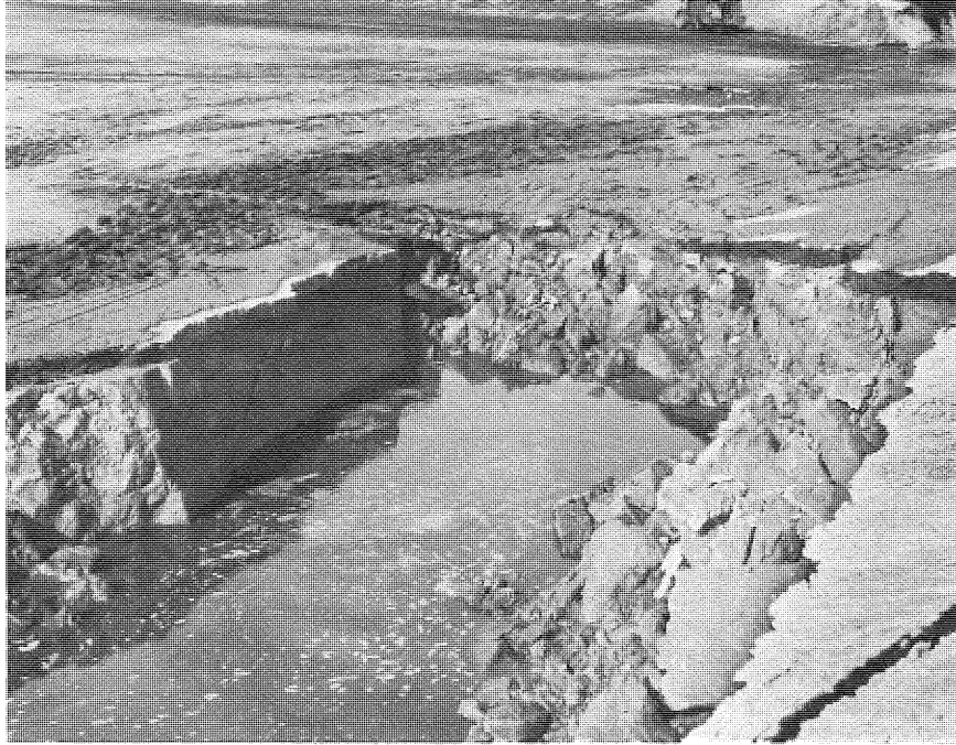
PHOTO 63. Ruptured lining near drainage inspection chamber, December 16, 1963.
