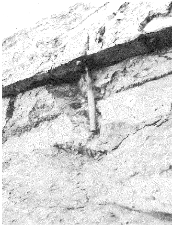
PHOTO 23. Close-up of slip-bed showing the magnitude of movement, which measured a maximum of 0.43 foot.
