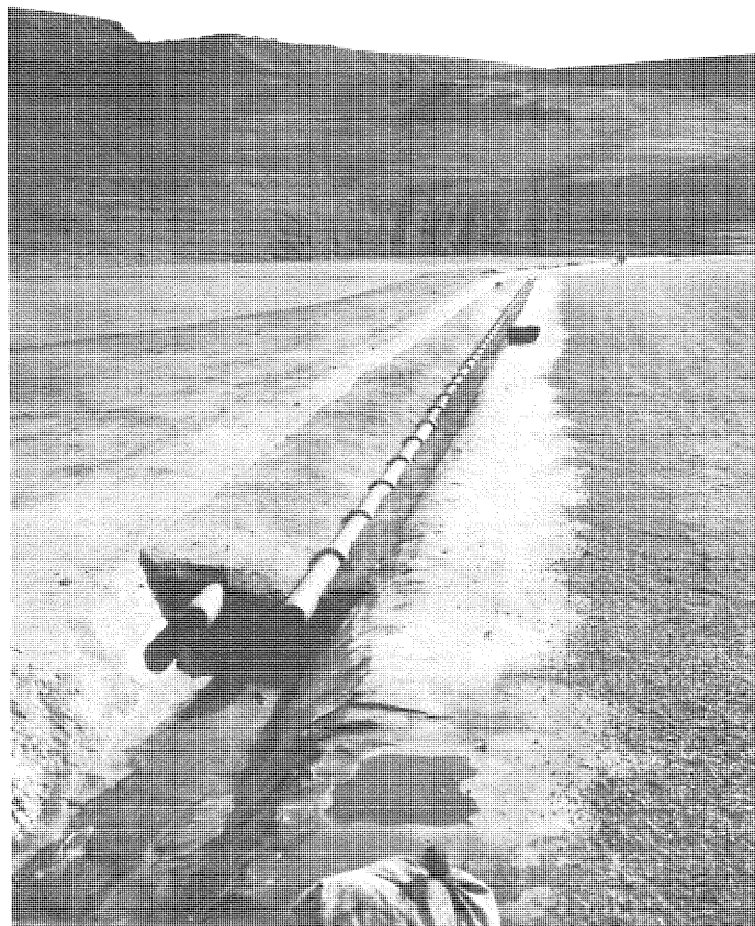
PHOTO 37. Installation of 4-inch tile drains. Note one line completely encased in concrete and other with open joints on top.
