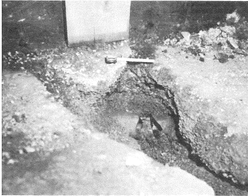
PHOTOS 85. Broken 4-inch clay tile drain in Excavation No. 8. Faces of break were coated with a calcium carbonate deposit.
