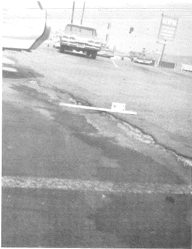
PHOTO 53. Earthcrack 2. Looking north across restaurant parking lot near southwest corner of Stocker Street and La Brea Avenue. Maximum vertical displacement 2 inches. Opening 1 inch.
