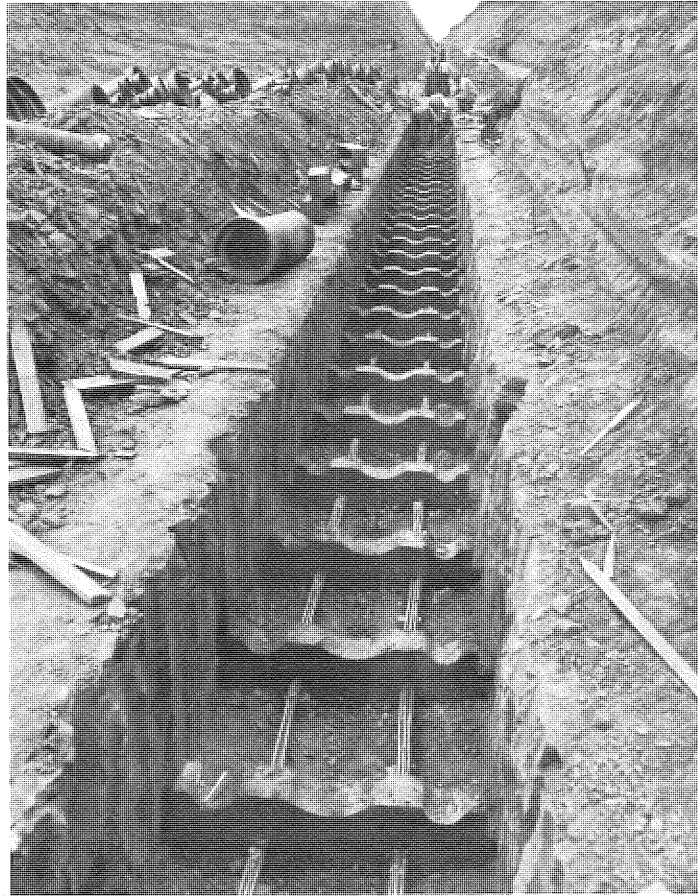
PHOTO 24. Foundation drainage details—Cradles for 4-inch and 12-inch tile and copper tubing for settlement measuring devices.
