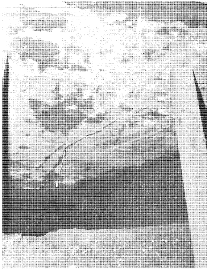
PHOTO 79. Break in north wall of drainage inspection chamber at Station 0+89 as exposed in Excavation No. 7B. Break closes to hairline crack at top.
