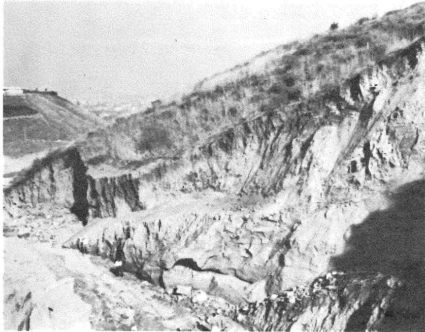
PHOTO 70. Landslide plane exposed in east side of breach, believed to be part of slide encountered during construction of dam.
