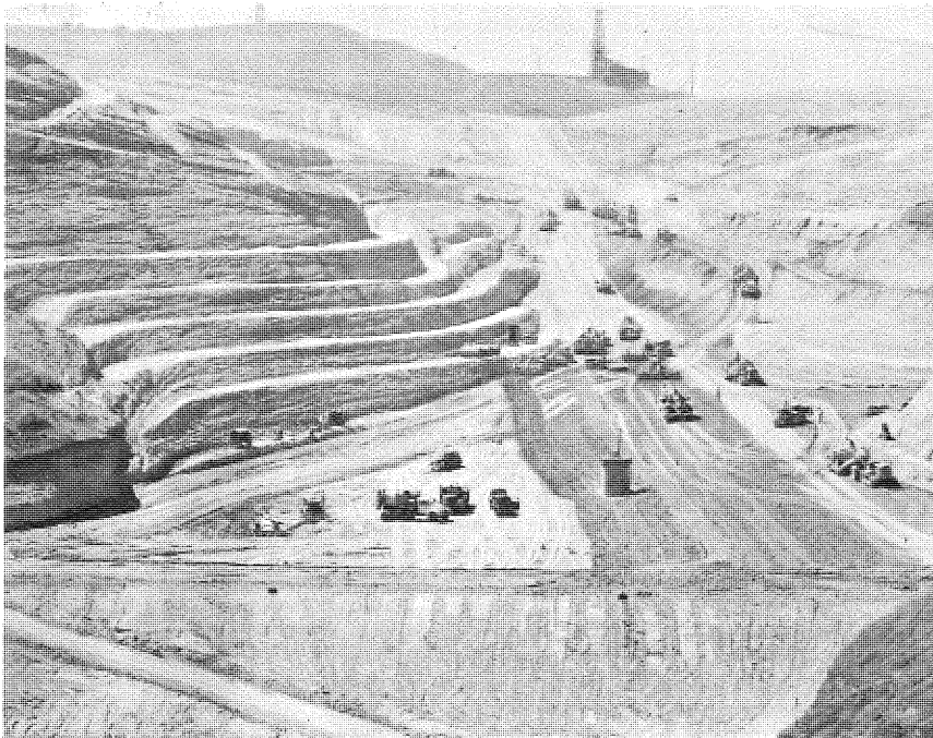
PHOTO 27. Looking upstream, showing benching on east abutment of main dam, Manhole A, 42-inch spillway pipe and catch basin on Elevation 340 berm.
