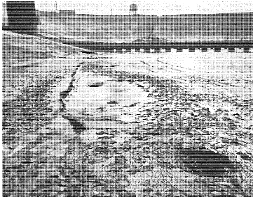
PHOTO 64. Sink holes and collapse features west of surface expression of Fault 1 along east side of reservoir.
