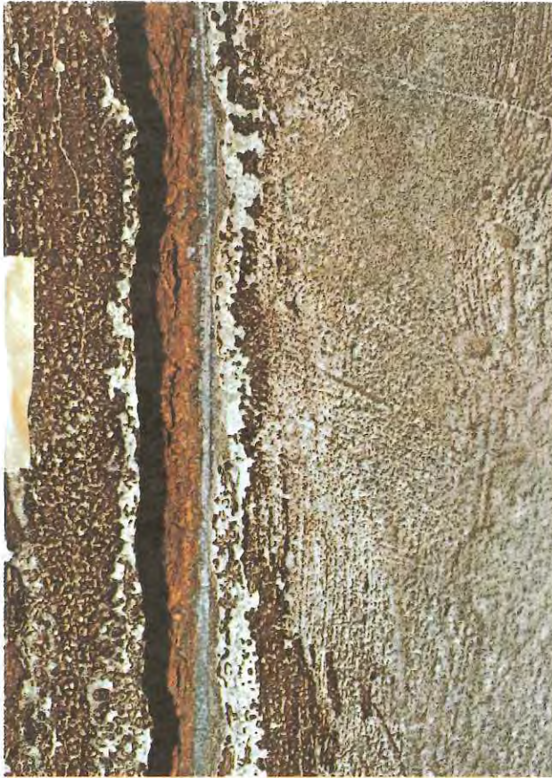
PHOTO 90. Interior of circulator connector conduit, showing corrosion of steel bell ring at a joint where the cement mortar lining separated. Blue line is uncorroded steel recently exposed.
