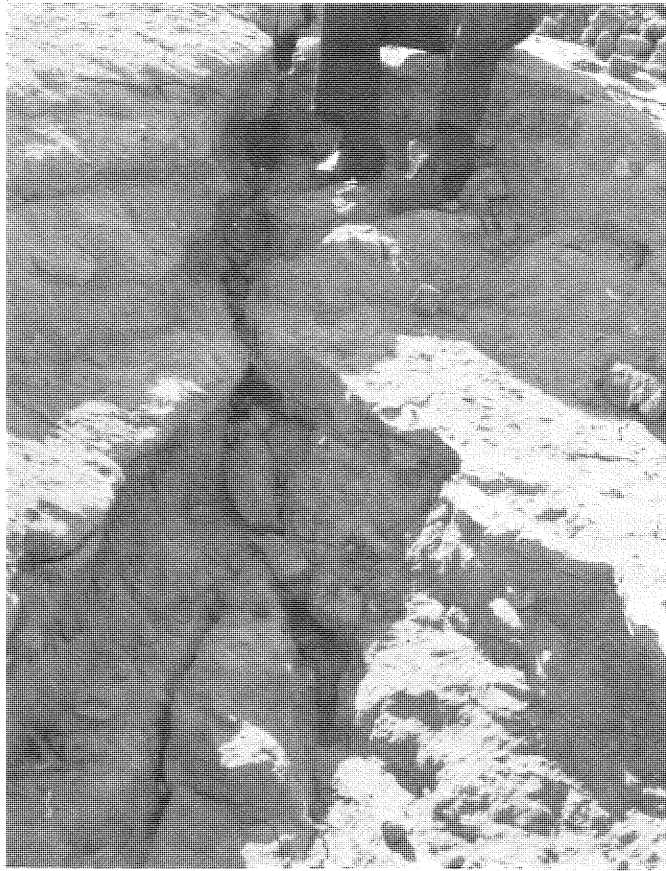
PHOTO 74. Scour and cracking in main dam downstream from 340 berm, January 4, 1964.
