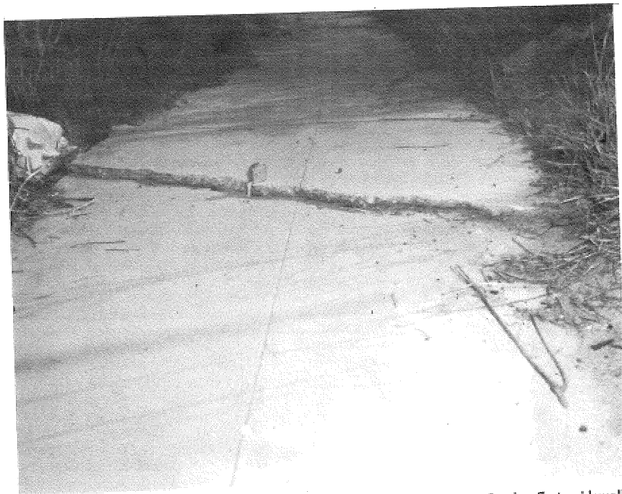
PHOTO 56. Earthcrack 6 near Don Miguel and Don Lorenzo Drives. Crack offsets sidewalk about 1 inch.
