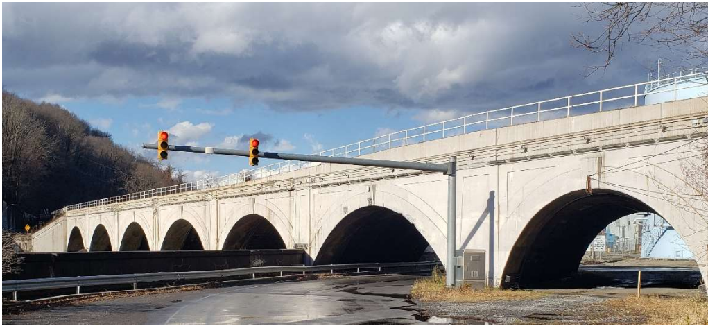
Figure 36: The seven-arched Stone Bridge, Johnstown. The Pennsylvania Railroad later covered its upstream face with concrete during a widening project. Source: Author.
